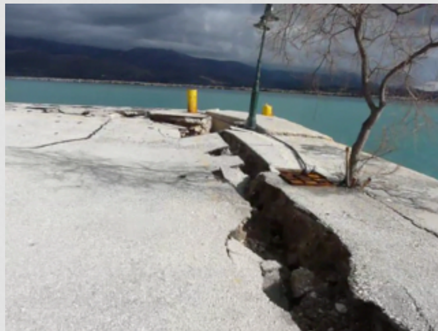
Figure 7. Liquefaction-induced damages in the quay in Lixouri (7/02/2014)
